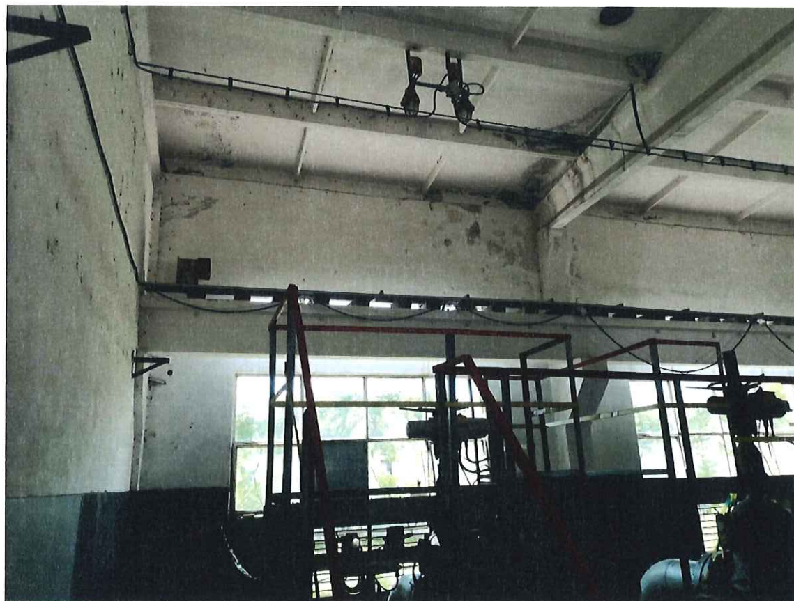
DETALIU INFILTRATIE IN ACOPERIS
