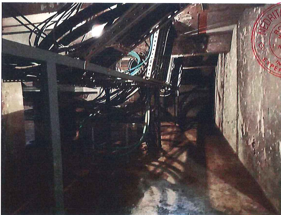
SUBSOL TEHNIC - CORP DISTRIBUTOR C – INFILTRATII PRIN PERETI SI PARDOSEALA.
