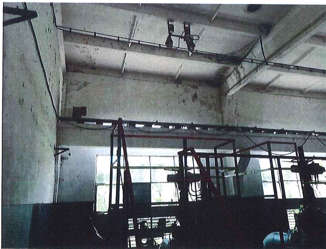
DETALIU INFILTRATIE IN ACOPERIS
